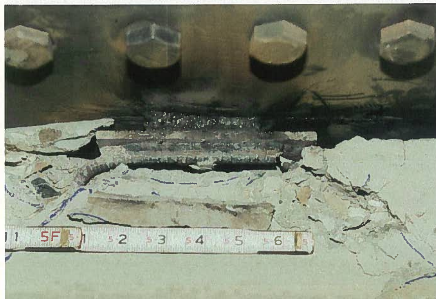
Fig. 25. Typical crack pattern at failure for specimens with a hairpin connector.
