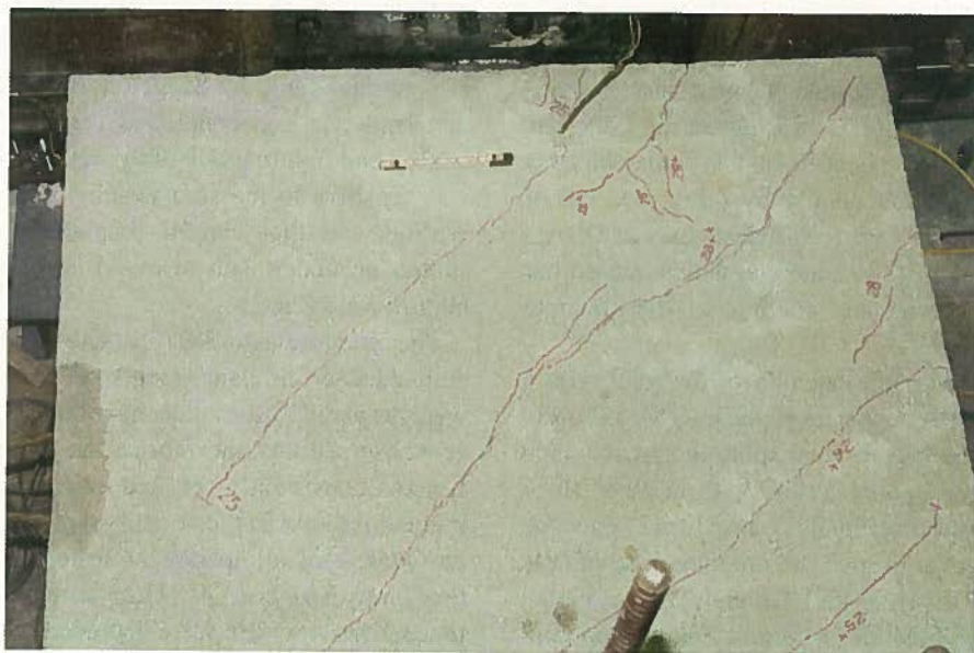
Fig. 27. Diagonal cracks in panels with a structural tee connector.
