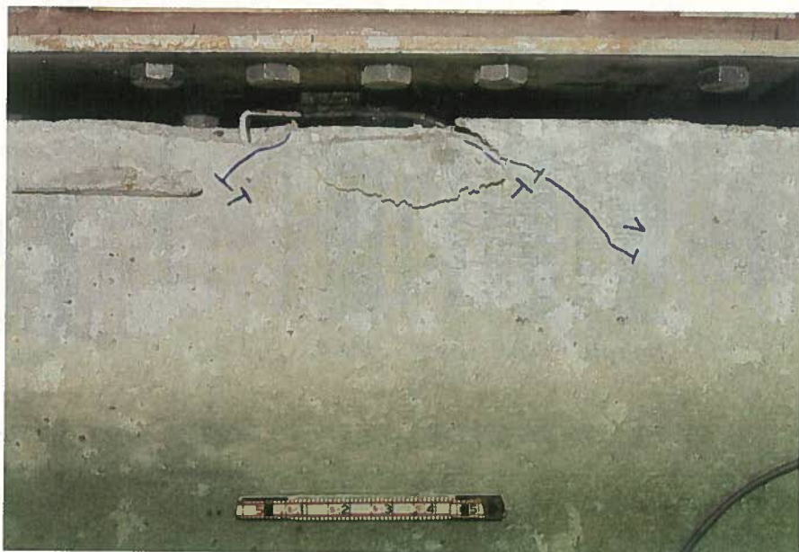
Fig. 26. Typical crack pattern at failure of specimen with a bent wing connector.
